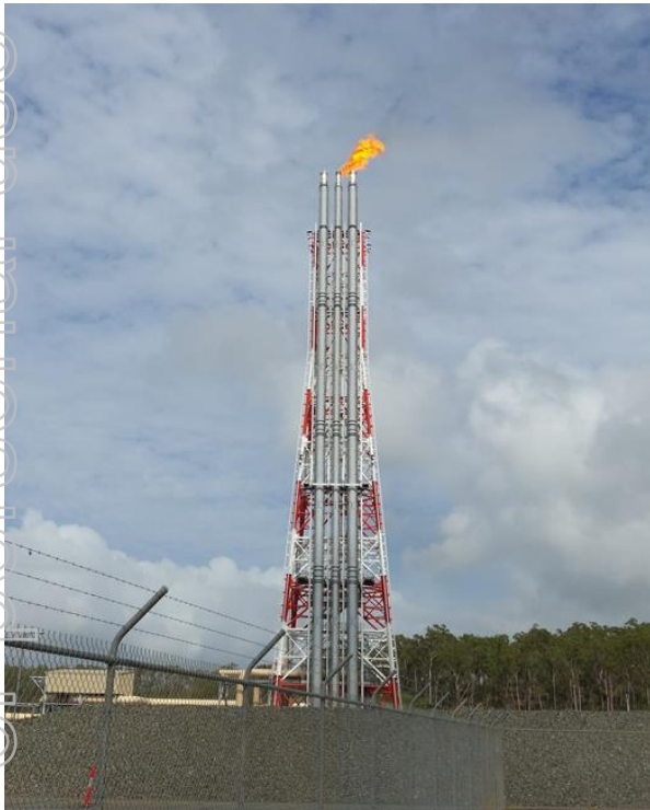
GLNG flare stack, Curtis Island, March 2015
