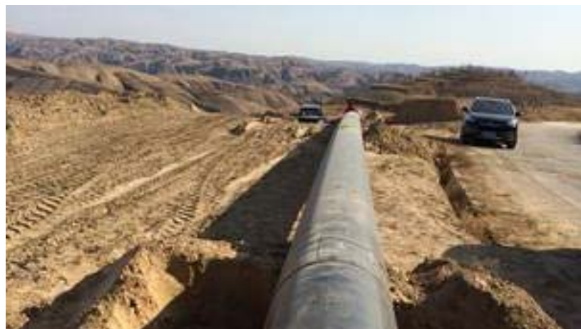
Third party Linxing Spur Line >100 MMscf/d capacity
