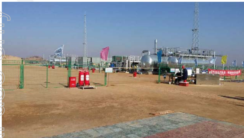
Sanjiaobei Central Gathering facilities commissioned
