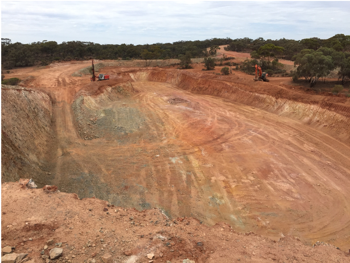
Figure 2: Jackorite open pit ready for drill and blast ahead of ore mark-up (5 January 2016)
