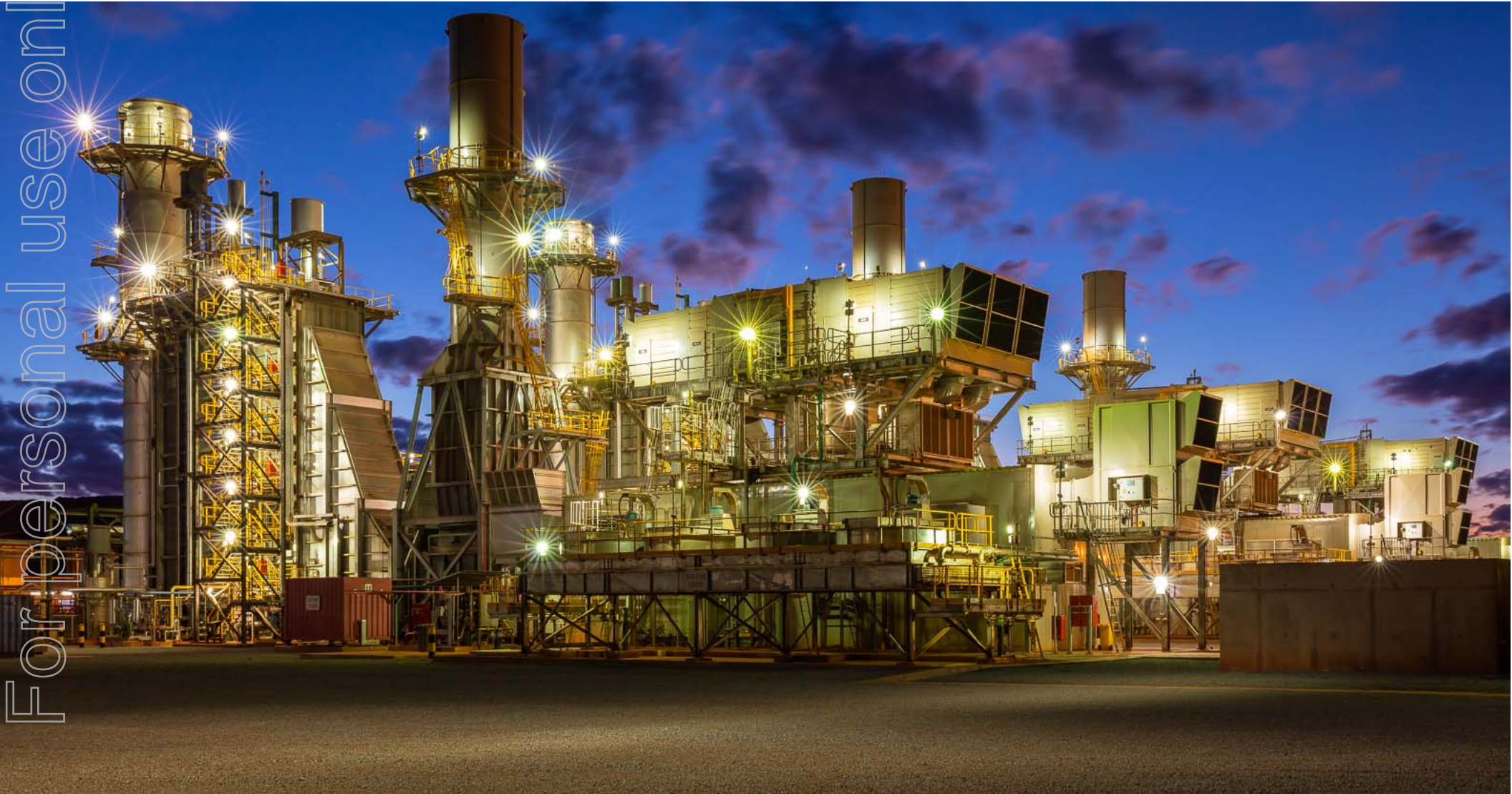
RCR Proprietary Heat Recovery Steam Generators, at BHP Billiton's Yarnima Power Station, WA
