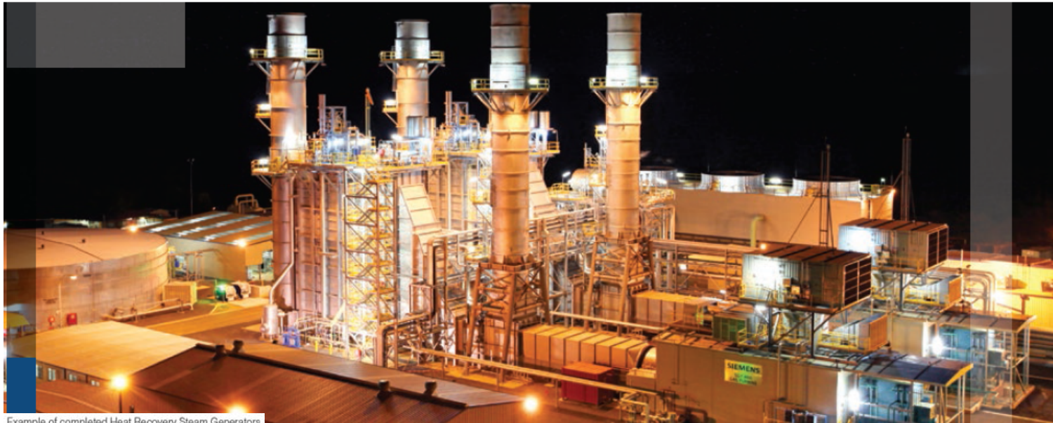
Example of completed Heat Recovery Steam Generators
