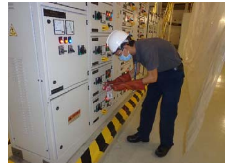
RCR Facilities Management works for Intel, Vietnam
