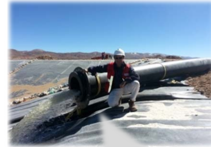
Aug 2013: First Brine pumping.
