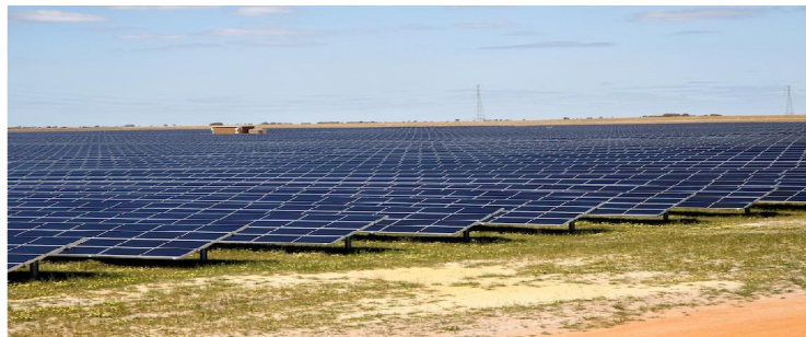
Royalla Solar Farm
