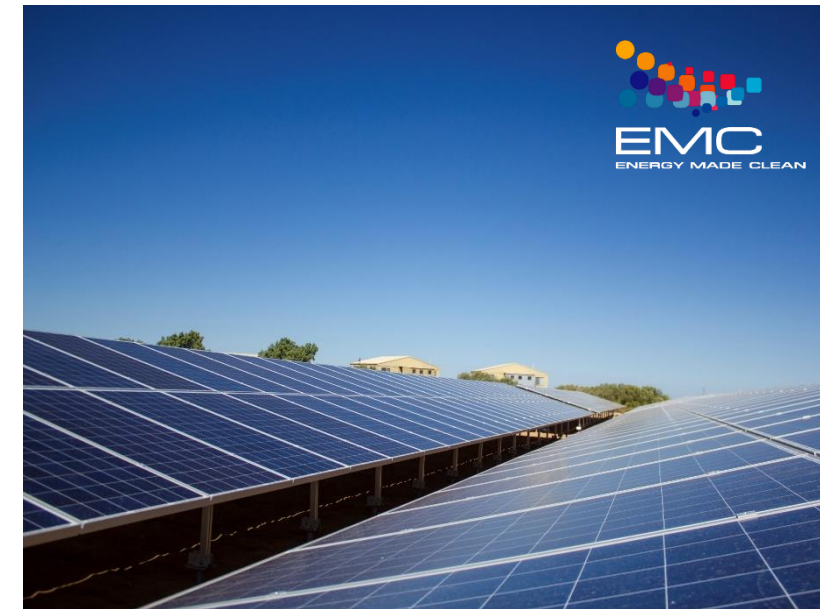
Remote monitored and controlled 100 kW PV /110 kVA Diesel/ 64 kWh battery project in outback Australia
