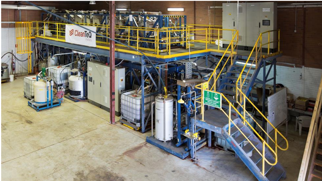
Figure 10: Clean TeQ's proprietary Resin-In-Pulp (cRIP) process demonstration plant, which can be used for production of NiSO 4 and CoSO 4 samples for customer testing
