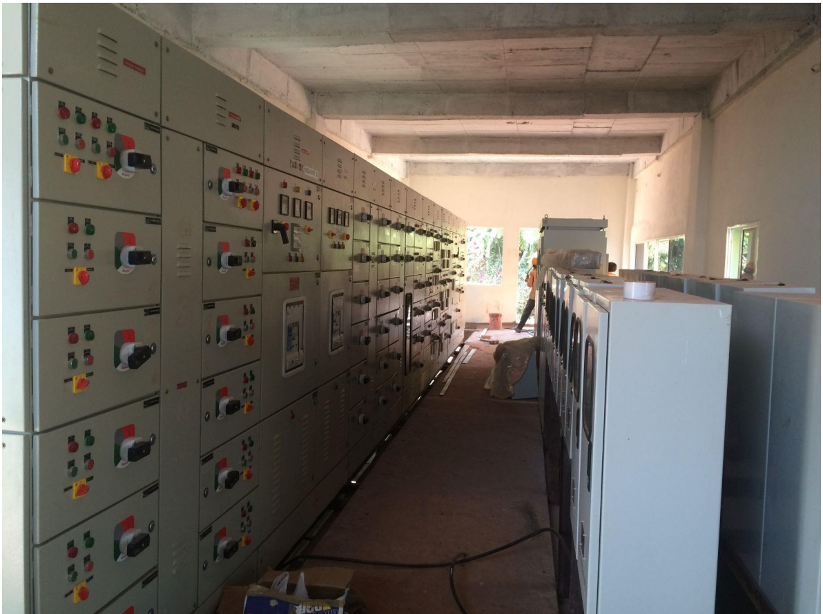
Internal Control Room Testing
