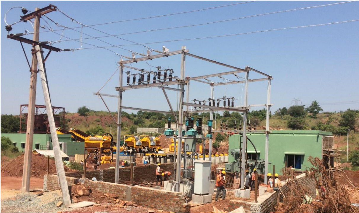
Switchyard to Main Transformer
