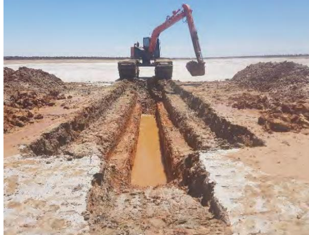
Photo: Trench excavation at Lake Wells 1 Significant trenching required to access low grade brines
