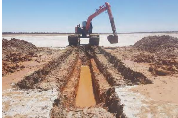
Photo: Trench excavation at Lake Wells 1 Significant trenching required to access low grade brines
