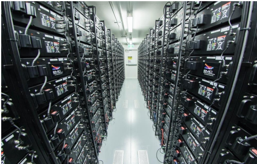
Utility scale battery energy storage system (BESS) designed and delivered by Carnegie's Energy Made Clean subsidiary for the Western Australian State Government owned energy utility, Synergy.
