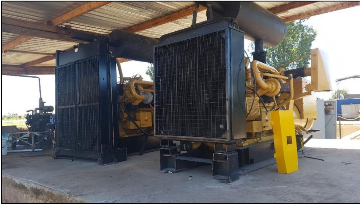
Figure 5 – Newly relocated Caterpillar generators.
