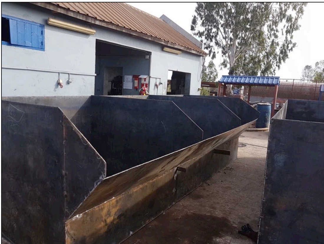
Figure 3 – Newly fabricated floatation cells.
