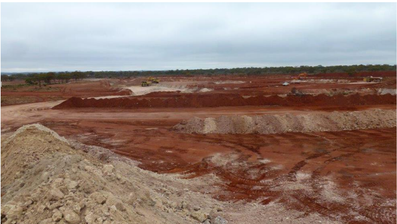
Initial mining and preparing the first bench at Penny's Find Gold Mine
