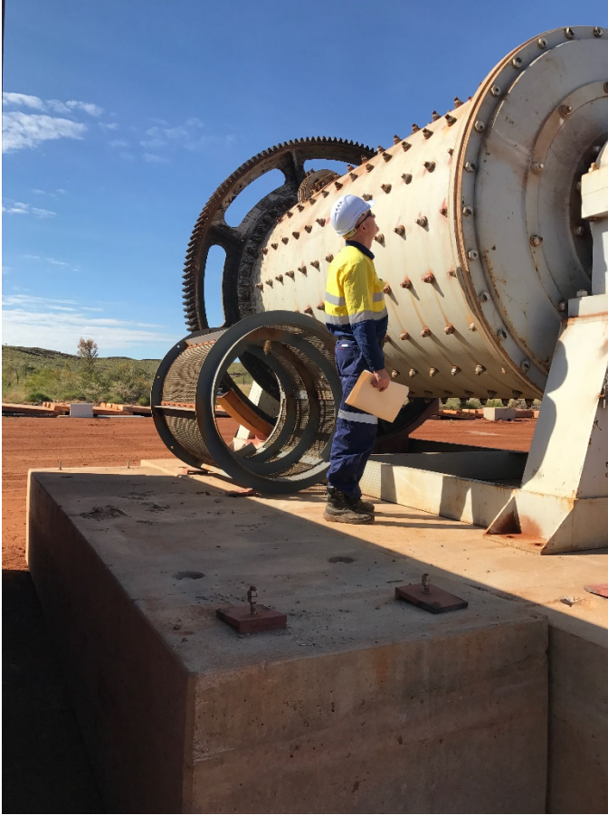
Figure 1: Ball Mill on foundations
