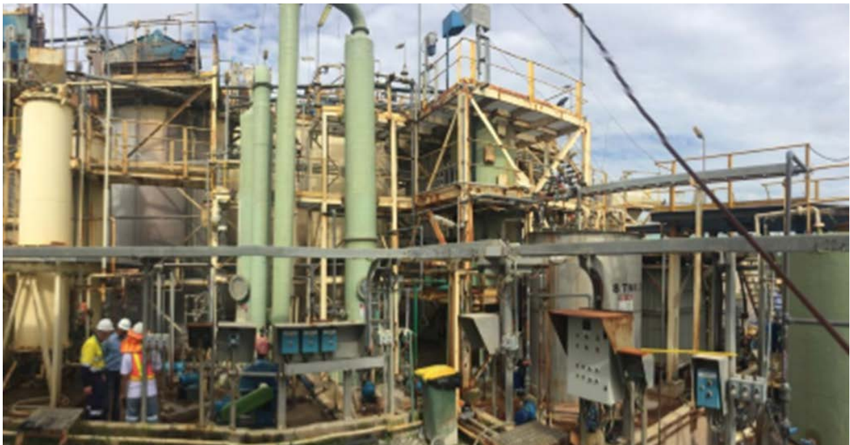
Figure 1 – Mirah Gold Mine cyanide recovery resin circuit.
