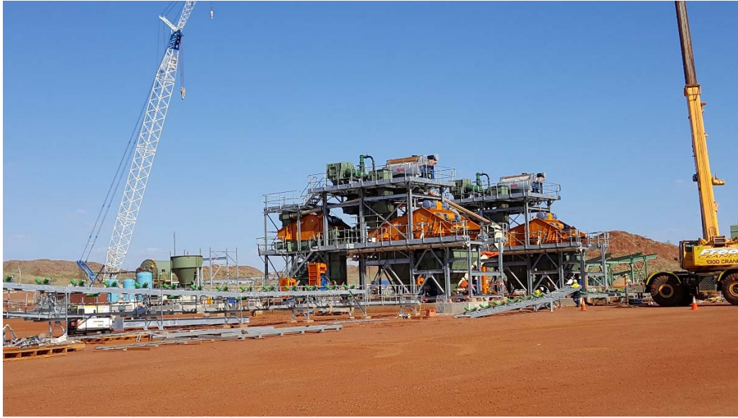
Dense Media Separation (DMS) modules 1 & 2
