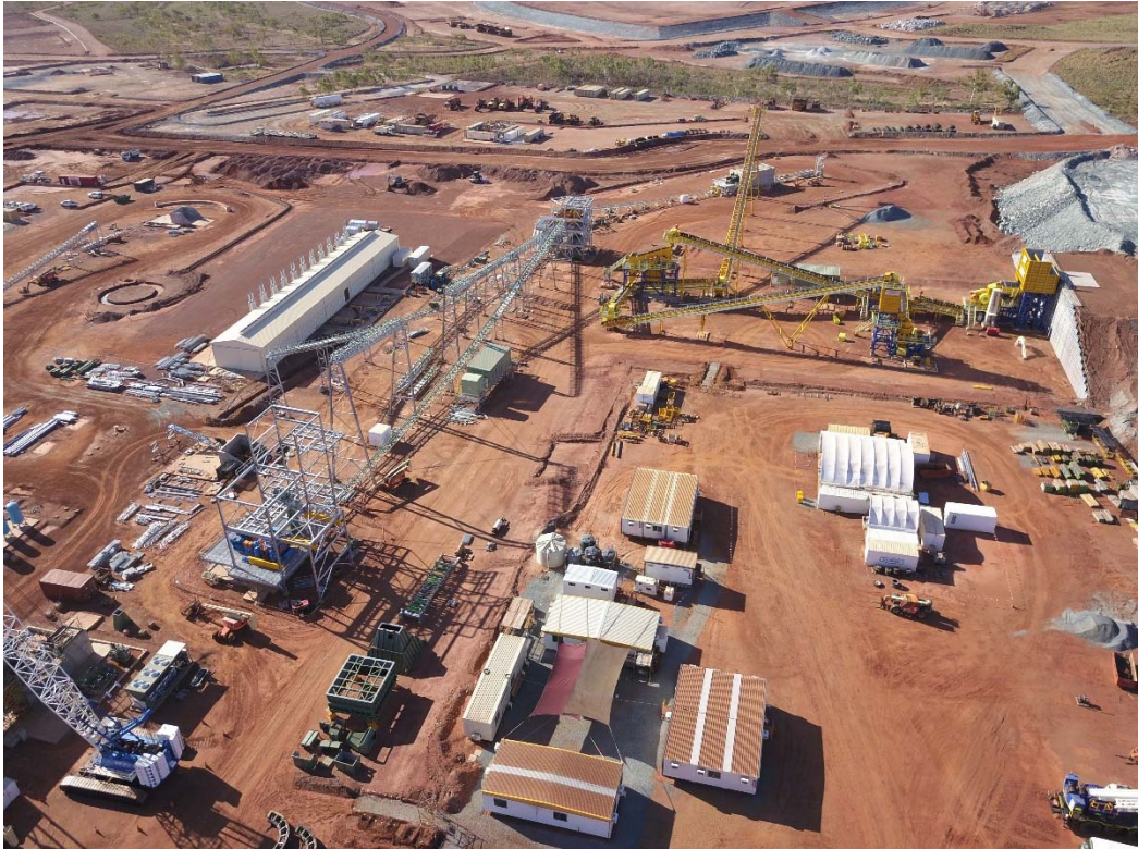
Drone photo taken from above the Process Plant control room
