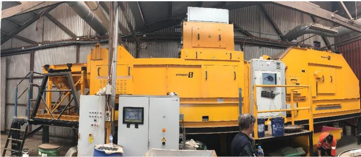
FIGURE 1 – STEINERT MULTI-SENSOR ORE SORTER AT NAGROM IN WESTERN AUSTRALIA
