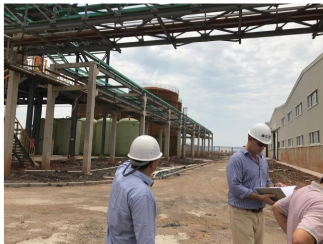
FIGURE 3: PLYMOUTH STAFF INSPECTING EXPANSION CONSTRUCTION ON A LITHIUM MICA PLANT IN CHINA
