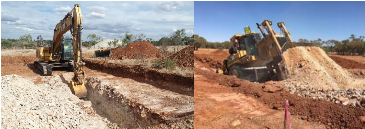
FIGURE: Ardmore mining trials; Excavator “free-digging” shallow phosphate rock (left), and dozer stripping shale overburden without the need for ripping (right).
