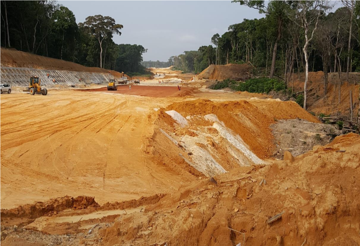
Figure 8: Earth works at the Kribi Port area for the new highway and rail
