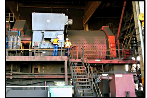
2.5MW Ball mill (photo taken at Rustenburg during independent inspection by METS).
