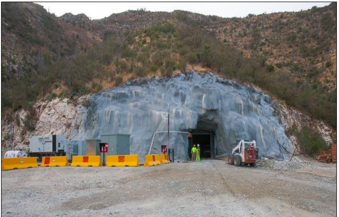
Figure 3 Refurbished 6400 Level portal with electric power infrastructure to left of portal. Note that generator shown in this photograph is currently off site
