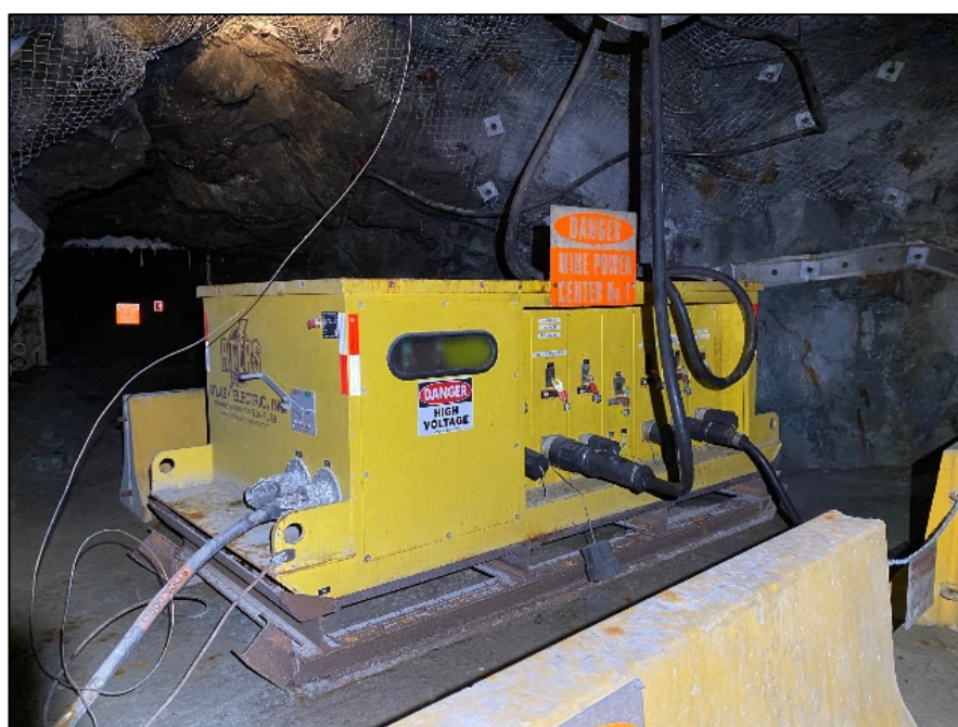
Underground electrical infrastructure
