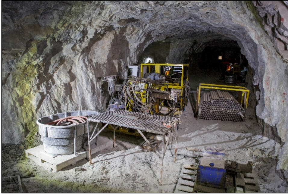
Underground electric drill rig and ancillary equipment
