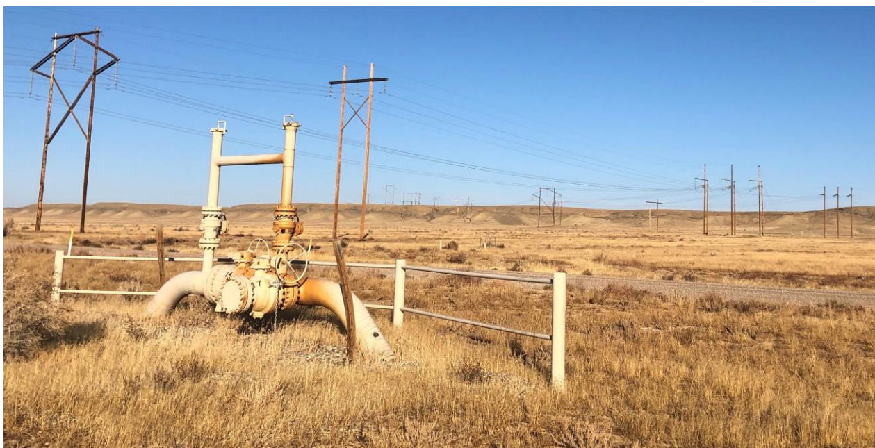
Figure 2: Picture of the Intersection of power transmission lines, natural gas lines and Blue Hills Rd.
