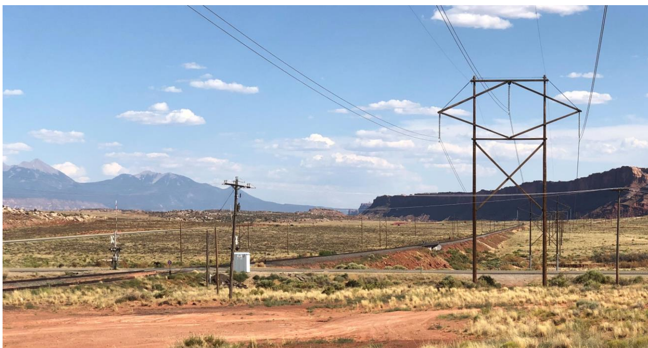
Figure 5: Picture of existing rail intersection with Deadhorse Point Rd. Highway 191 heading into Moab in background.
