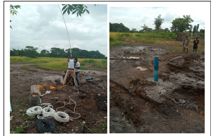
Casing the water well and lowering the pump (LHS). Newly drilled, cased and collared water well (RHS)
