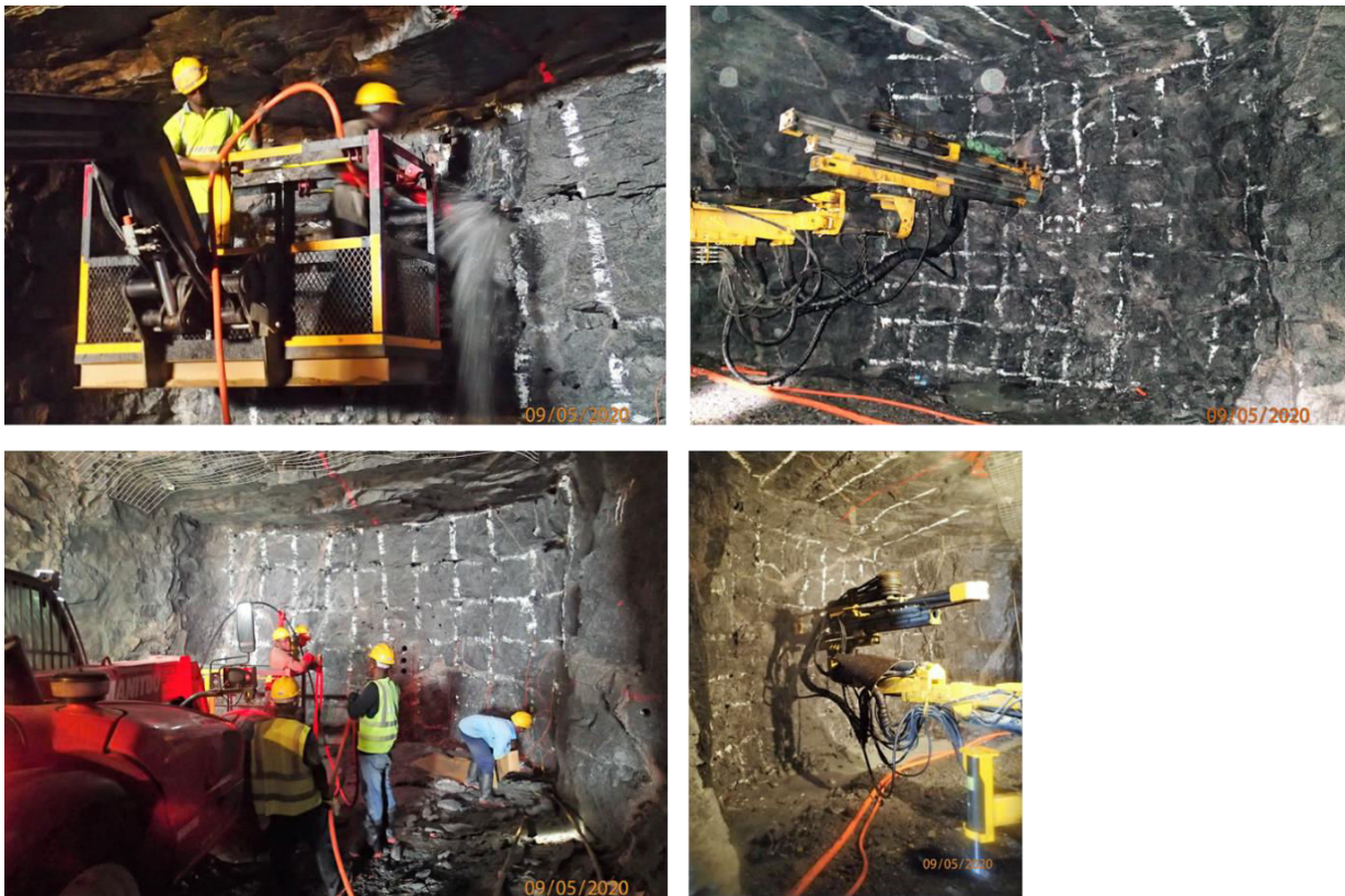
Figure 2: Underground drill and blast work underway. Top right and bottom right: drilling blast holes on a regular grid pattern; Top left: cleaning drilled holes; Bottom left: charging blast holes.
