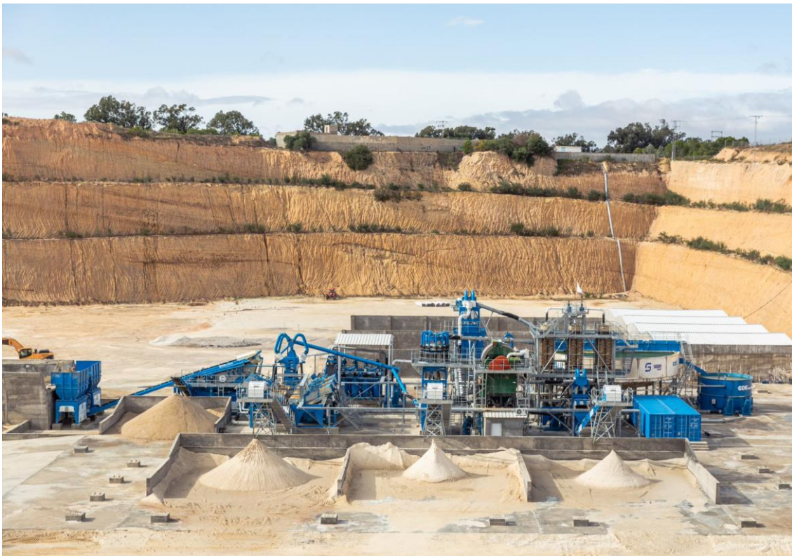
Figure 1: 200tph silica sand wash plant installed for SOMEVAM (Sebri Group) in Tunisia
