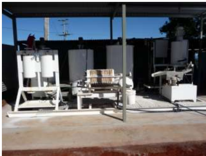
Figure 2: Upgraded Pilot Plant
