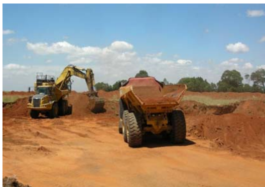
TMS Mining undertaking topsoil pre-stripping in the box-cut area at the Vlakvarkfontein Coal Mine
