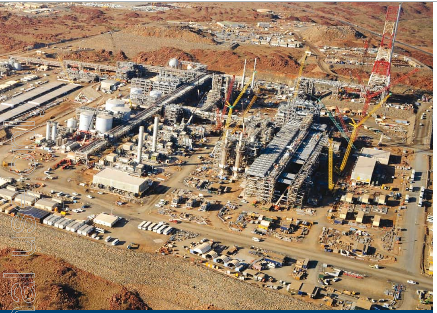
RCR provided all electrical and instrumentation works associated with the Pluto LNG Project main storage and condensate tanks and underground cable installation in the off plots and utilities areas. Photo courtesy of Woodside.
