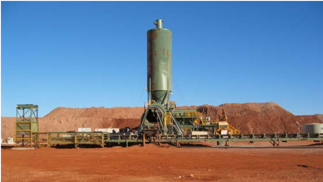
Agglomerator and Cement Silo
