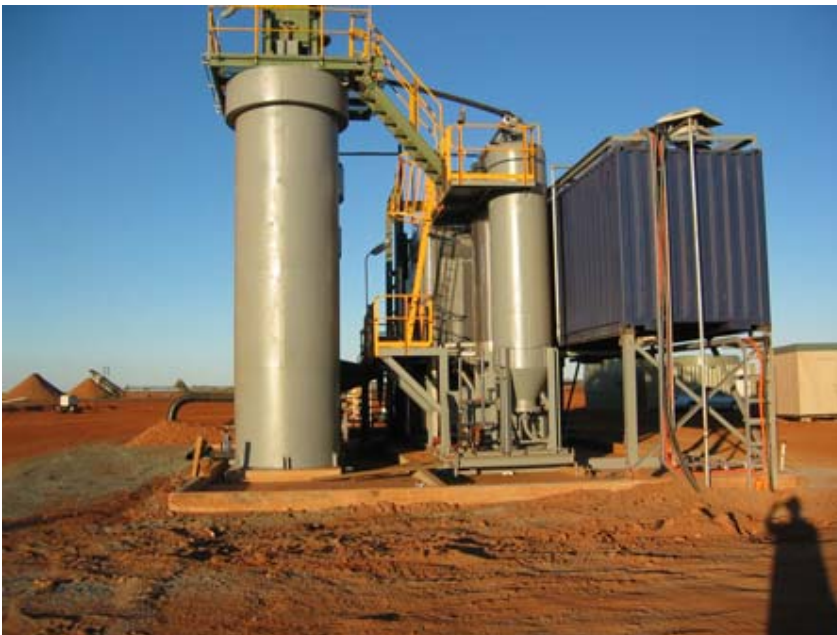
Carbon Tanks, Elution Column and Gold Room
