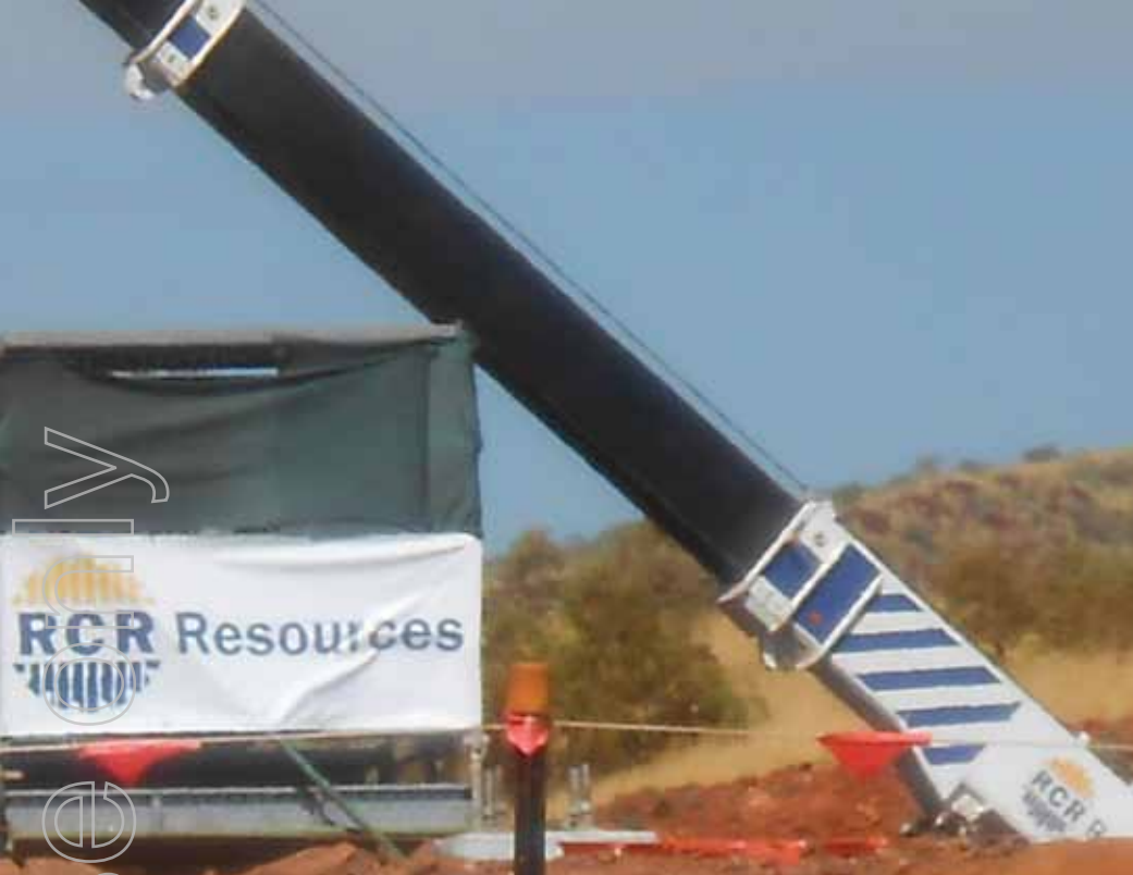
Crusher installation at Firetail Ore Processing Facility, part of Fortescue's Solomon operations
