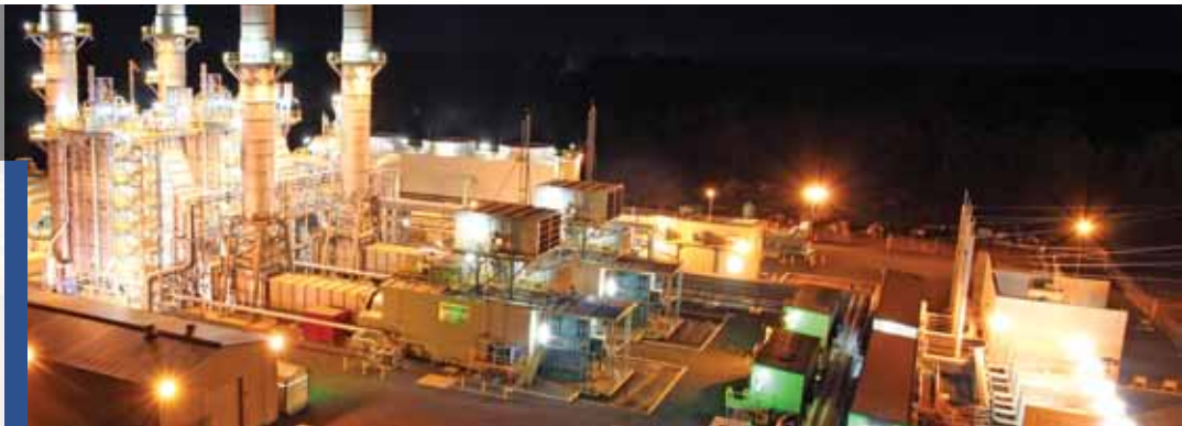
140MWe Combined Cycle Power Plant in Queensland
