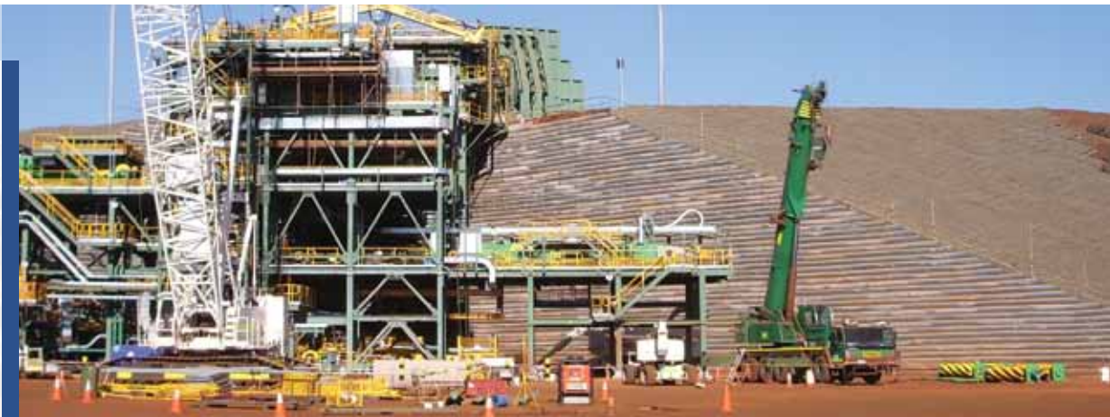
Primary Crushing and ROM bin, BHP Billiton RGP5 Yandi Operations
