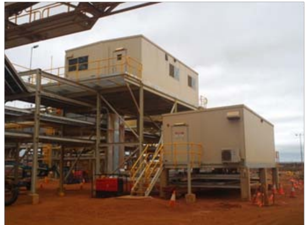
Switch Room & Control Room
