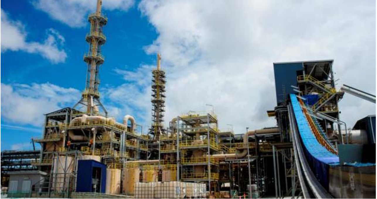
Concentrate loading and gas treatment
