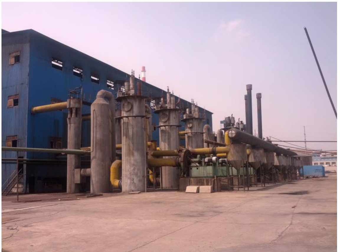
Gasifiers-Coal to Semi Coke and waste gas used to heat ovens
