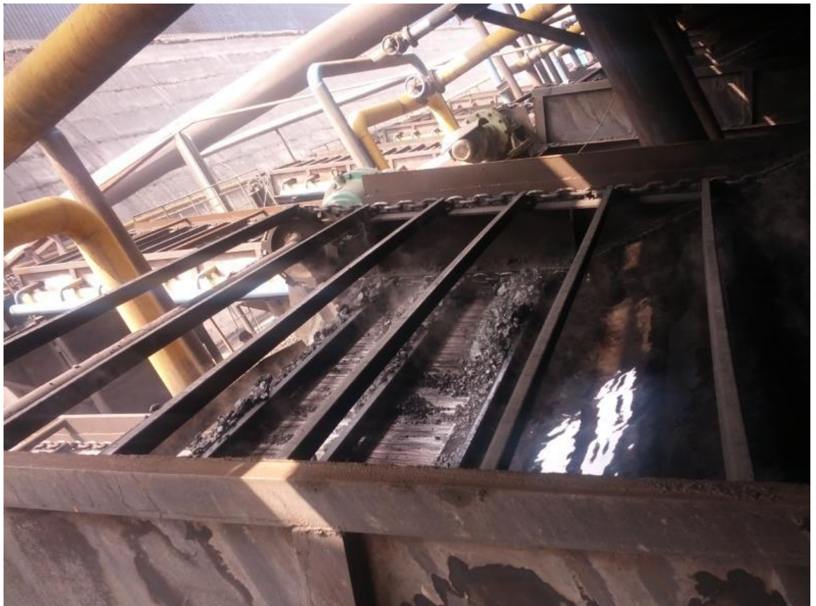
Discharging semi coke (2)
