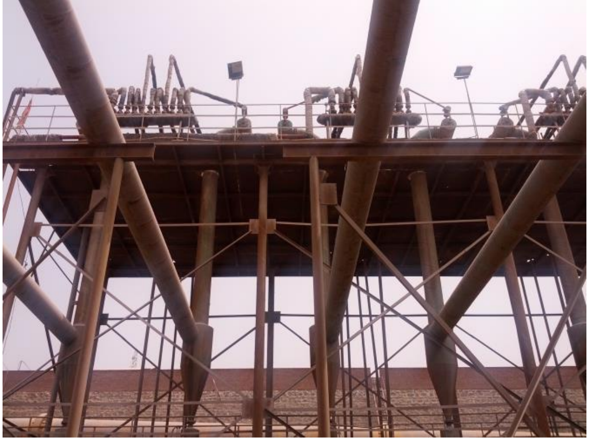
Steam powered vacuum system-steam from waste heat recovery system of rotary kiln
