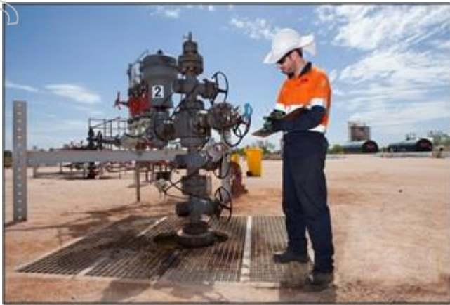
Ungani 2 well head and Buru Energy field operator
