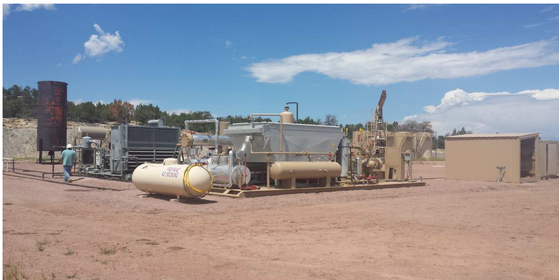
Austin's Pathfinder Gas Processing Plant. Fremont County, Colorado
