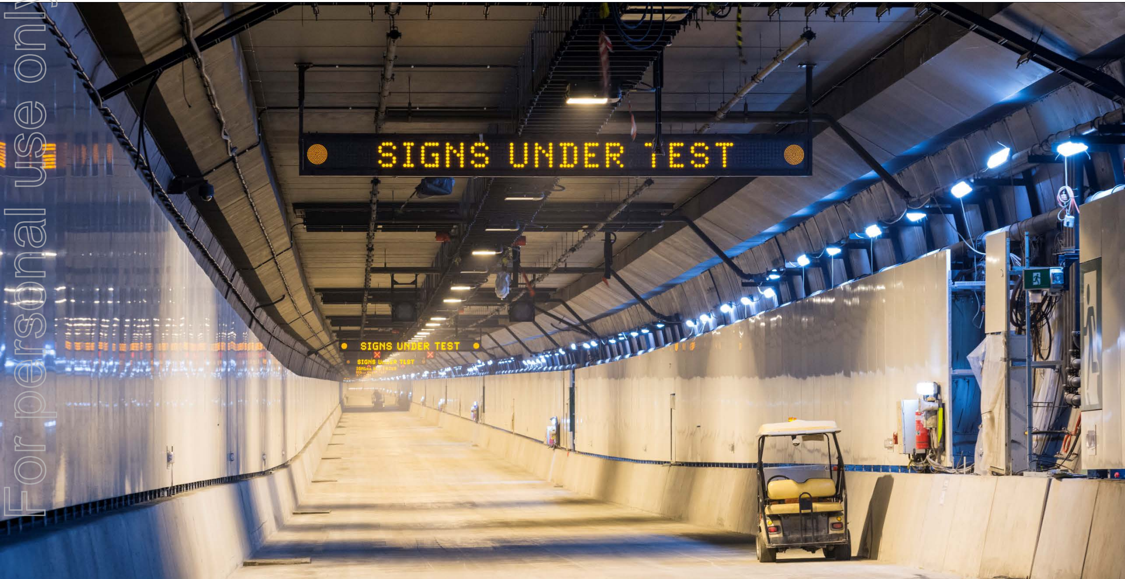
RCR delivered Mechanical & Electrical fit-out at Transcity JV's Legacy Way Tunnel, Brisbane, QLD
