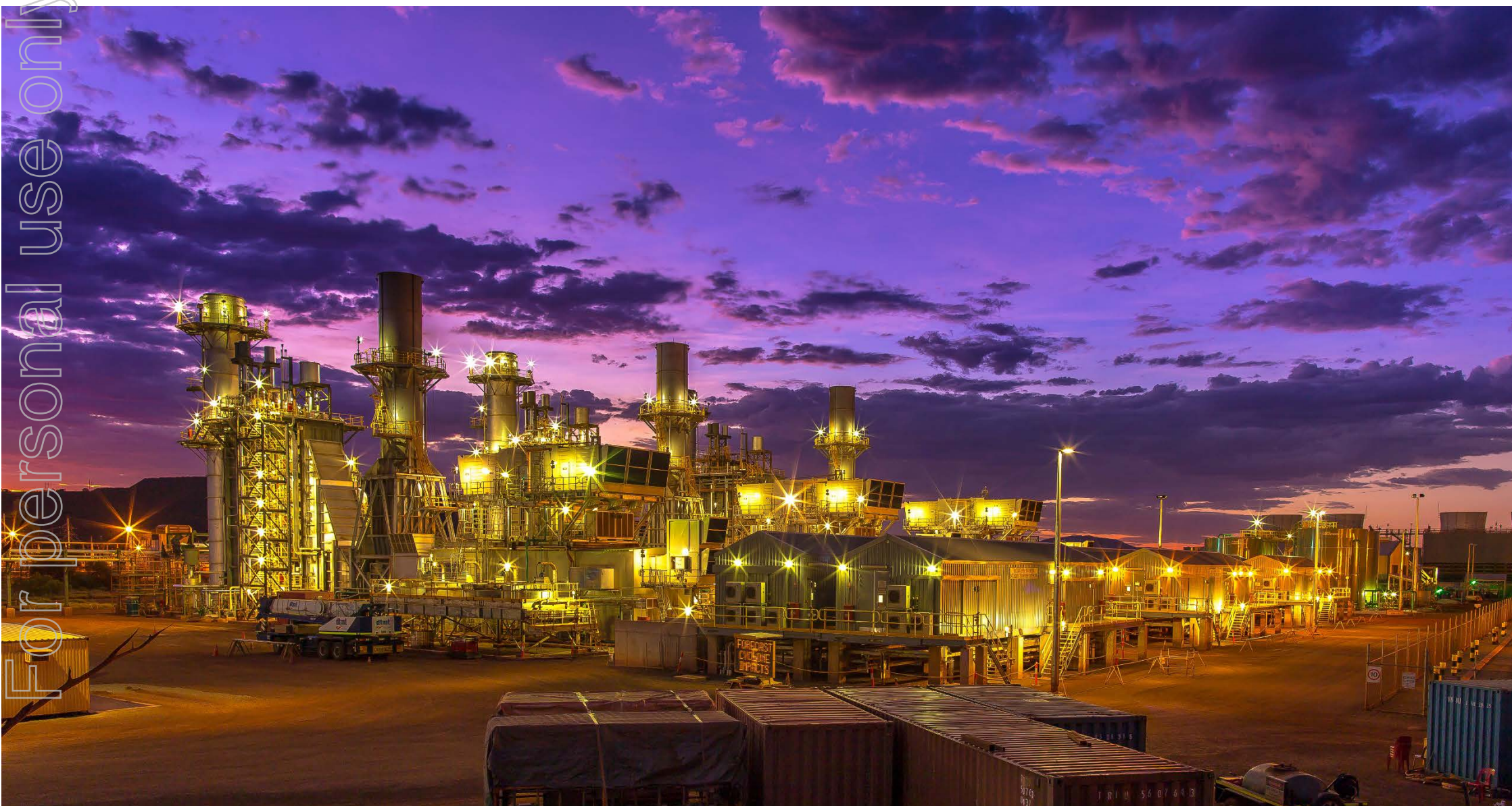
RCR Proprietary Heat Recovery Steam Generators, Yarnima Power Station, WA
