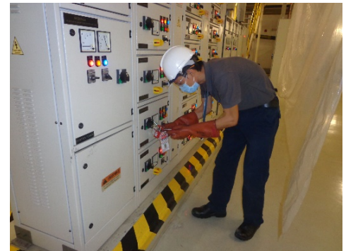
RCR Facilities Management works for Intel, Vietnam
