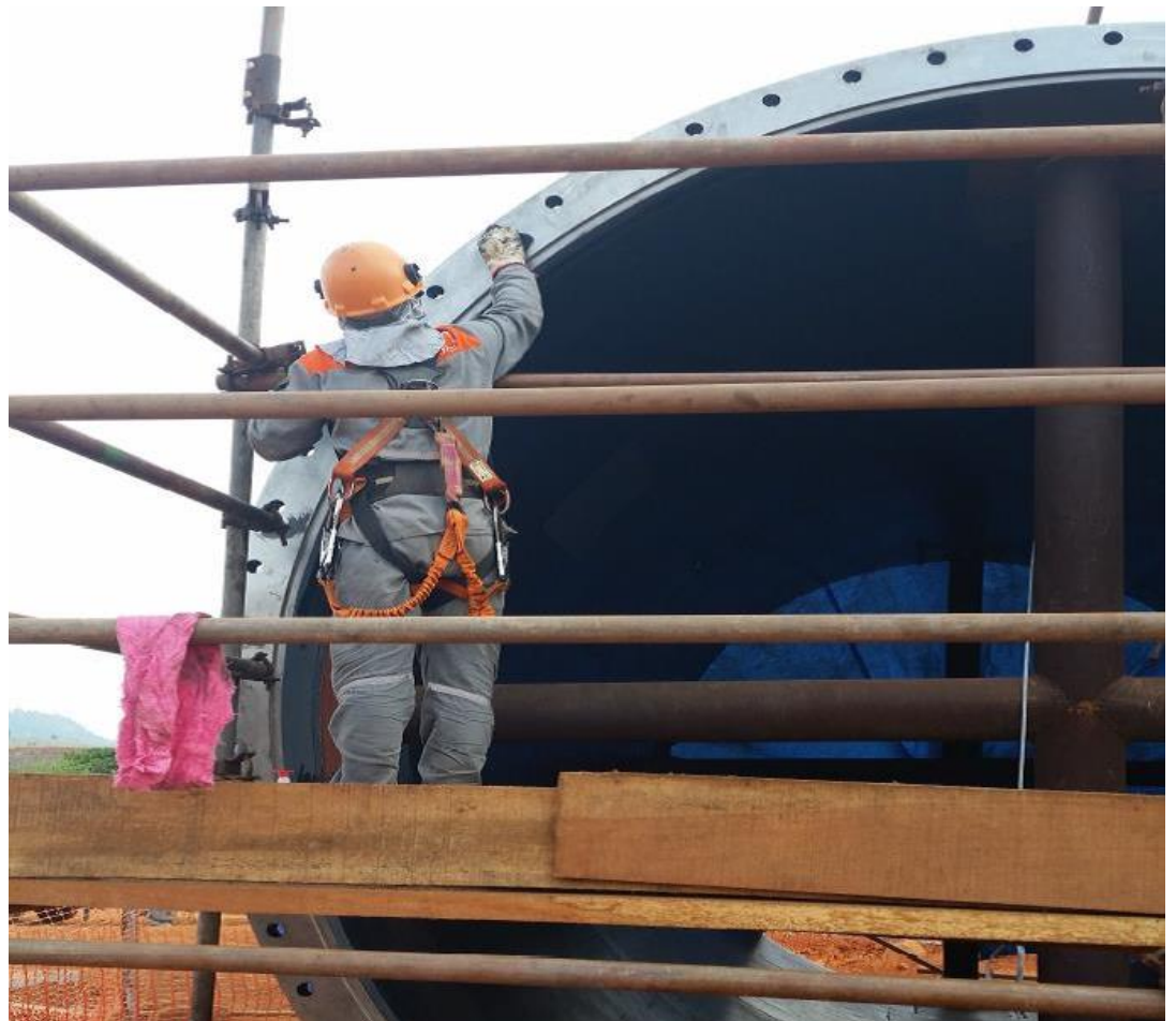
The 12'x24' Metso Ball Mill shell (flanges) being prepared for mounting of the trunnion heads
