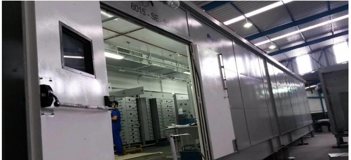
Flotation area electrical installation is facilitated by the use/delivery of pre-wired Motor Control Centers
