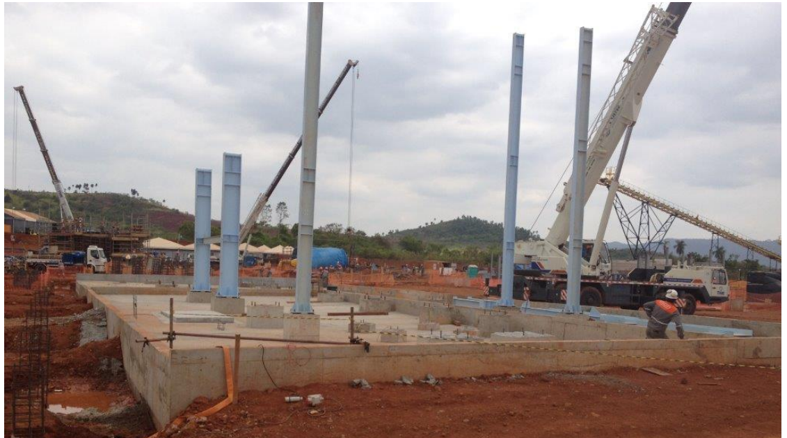
Flotation floor civils are sufficiently advanced to allow the start of structural steel which will support the float cells
