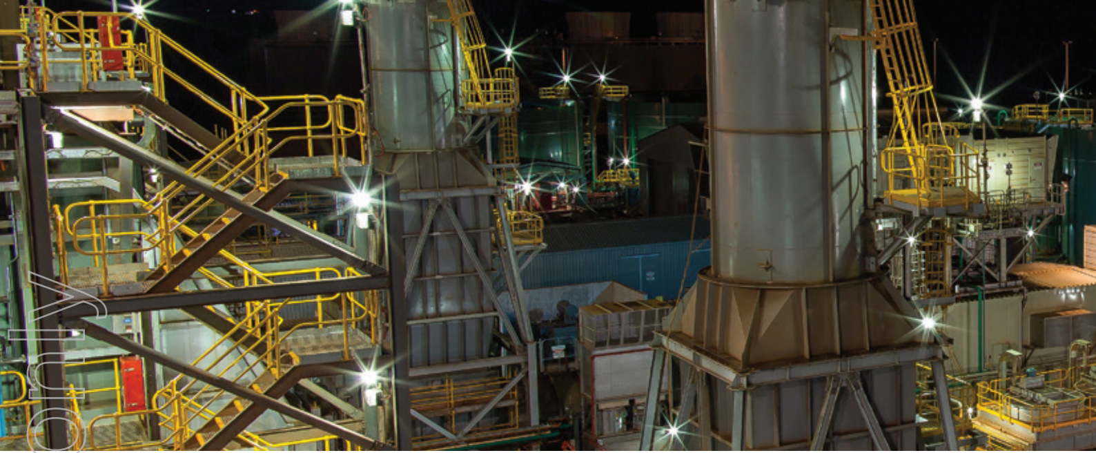
RCR Proprietary HRSG Technologies designed, supplied and installed at BHPB's Yarnima Power Plant, WA.
