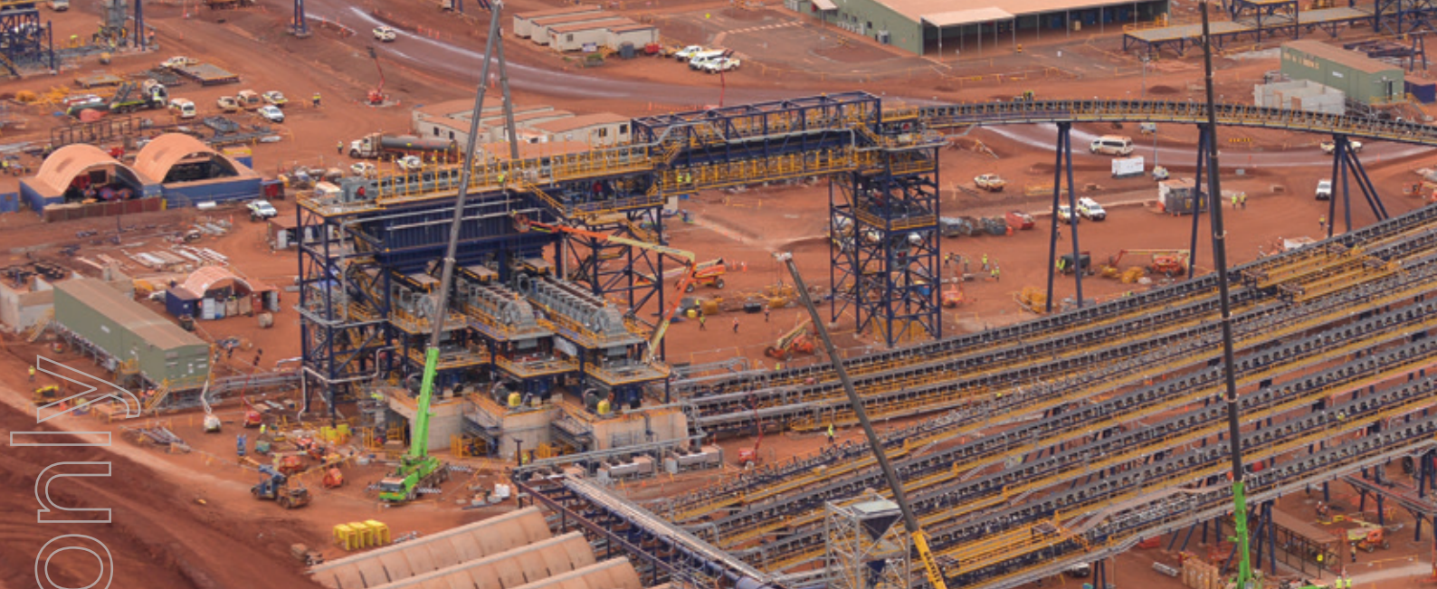
SMP and E&I works at the Roy Hill Iron Ore Project, WA.
