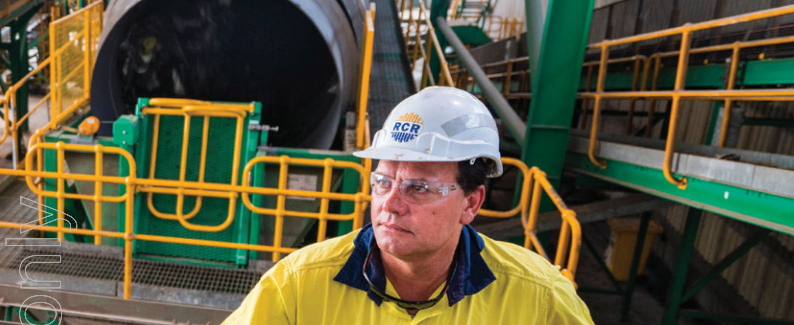
RCR fabrication, installation and E&I works for the Composter - Neerabup Treatment Plant, WA.
