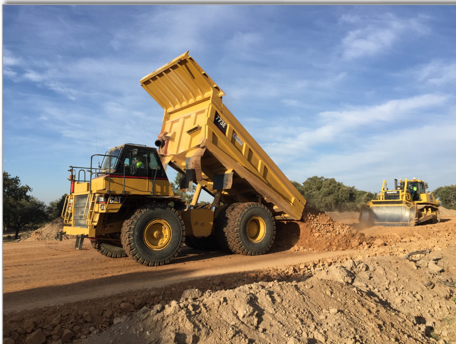
Mine contractors constructing the new 5 kilometre road at the Salamanca project in Western Spain
