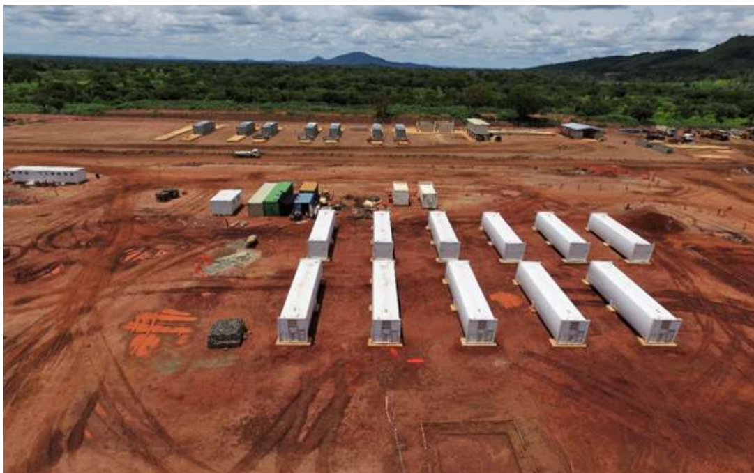
Figure 13 – Diesel fuel storage facility and power station (background)
