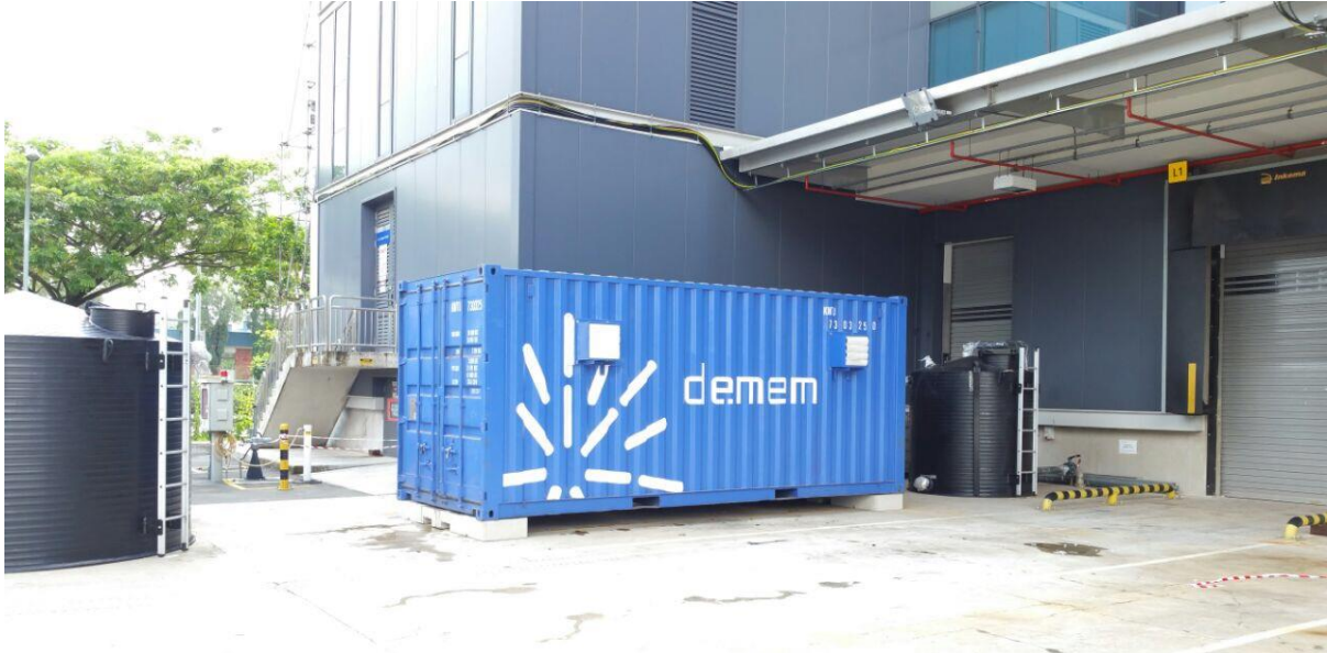
De.mem's containerised water treatment system on-site at a customer's factory
