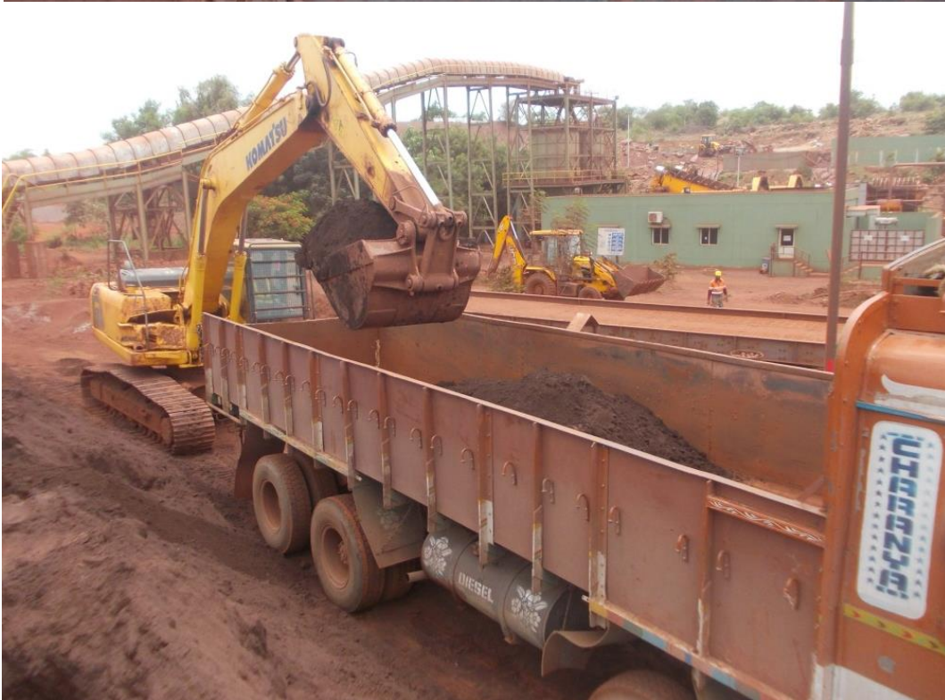
Loading and dispatch of the 60/61%Fe filter cake to Minera.
