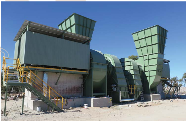
Ventilation Fans installed at Tritton Underground Mine over the new exhaust ventilation shaft
