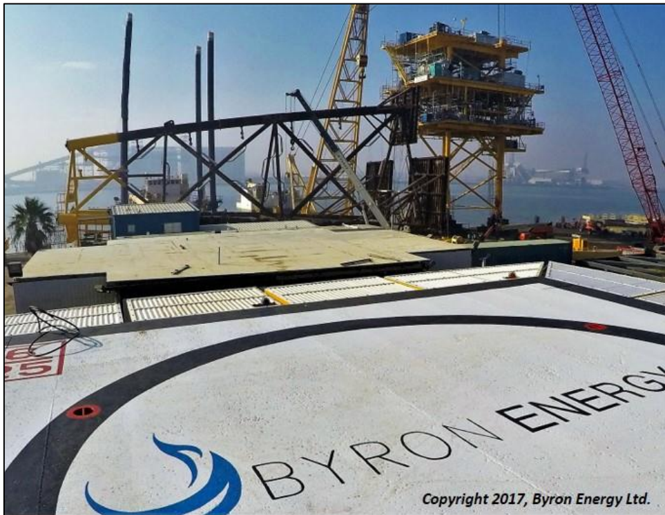
Byron Energy operated SM71 "F" helideck, jacket, and platform preparing for load-out. Galveston, Texas
