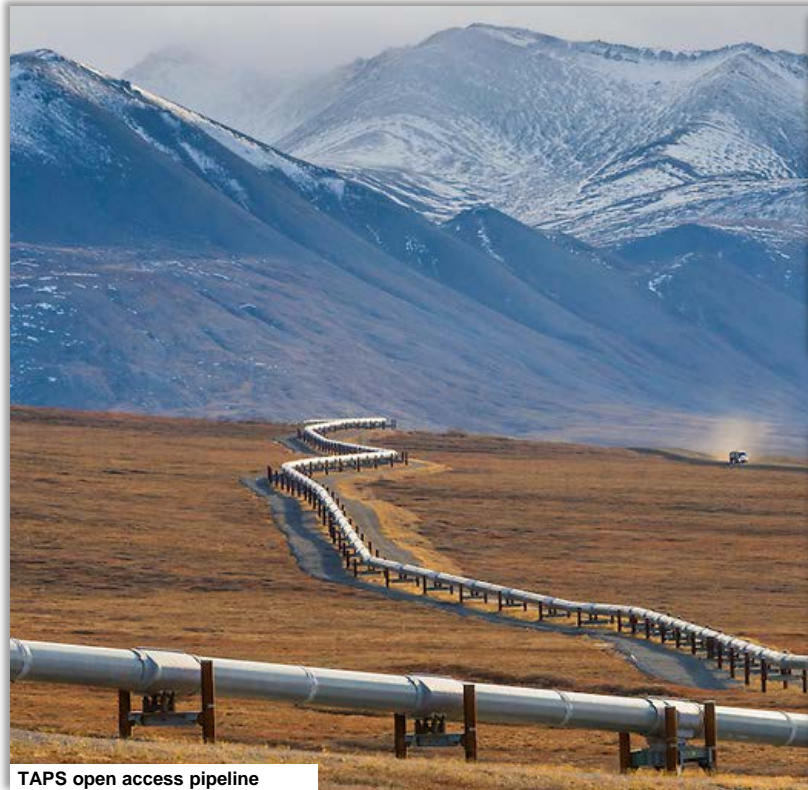
TAPS open access pipeline
