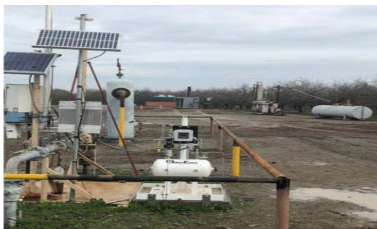
Dempsey 1-15 Natural Gas Sales Point
