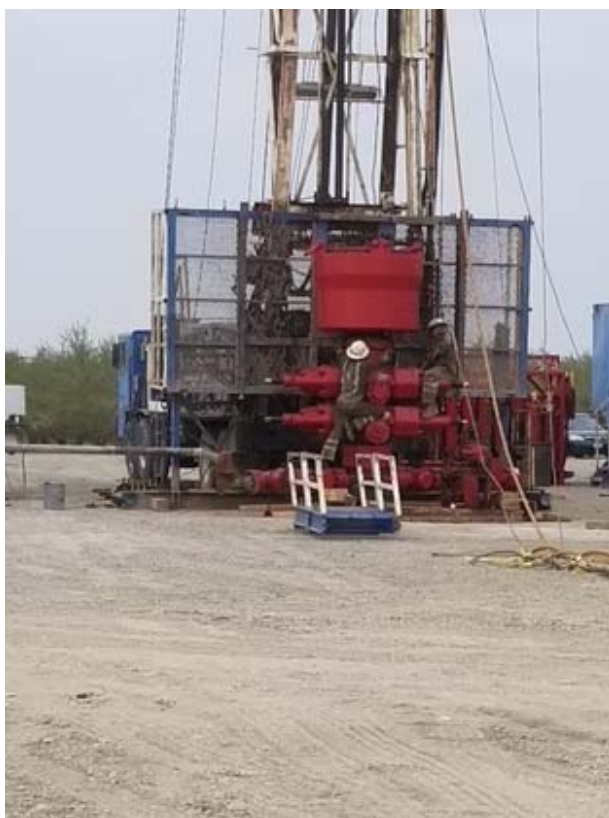
Dempsey Completion Rig featuring 10,000 psi BOP
