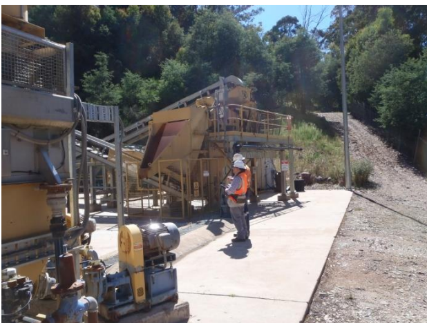
Photos 1 and 2: Inspection of plant for restart
