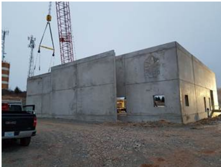
Figure 1: Construction of the medicinal cannabis production facility at the Mernova Medical site in Nova Scotia, Canada
