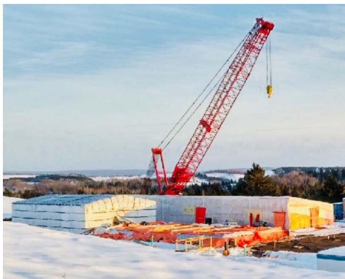
Figure 4: Construction of the medicinal cannabis production facility at the Mernova Medical site in Nova Scotia, Canada
